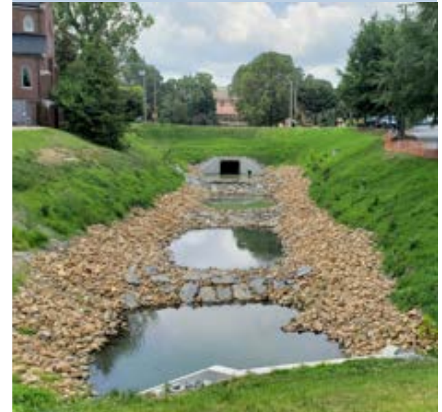
A regenerative stormwater conveyance system in Greenville, NC. Photo courtesy of WK Dickson & Co., Inc.
